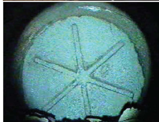
Plug within a 16-inch gas main
